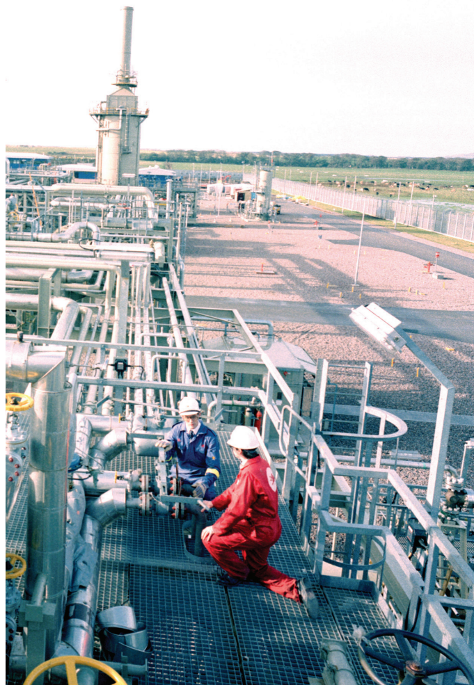
St. Fergus gas terminal, Scotland. ©Crown Copyright, Health and Safety Executive
