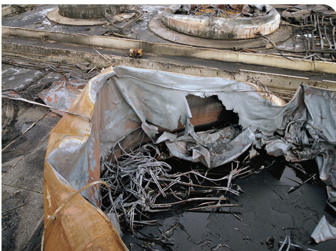
After effects of the fire at Buncefield oil storage facility. ©Crown Copyright, Health and Safety Executive
